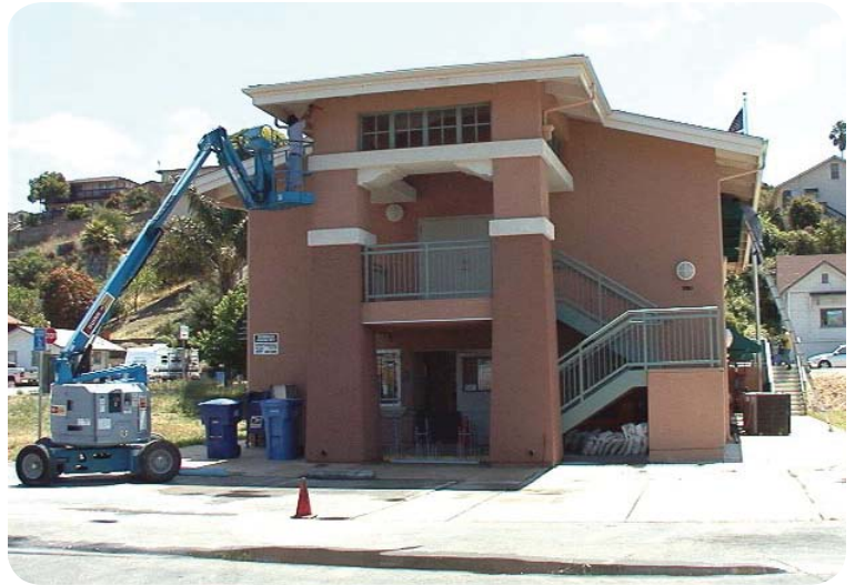
Netting installation on the Avila Beach Community Center and Post Office, photo courtesy of Stephanie Little
